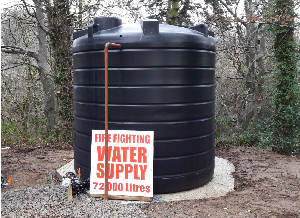
Photo 3 – Example of overground tank with signage
