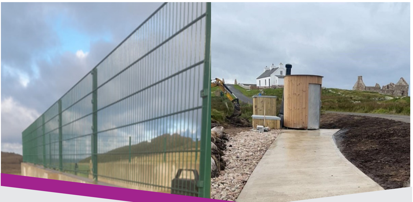
Tory Island Recycling Facility Fencing and Gola Island Dry Loo were completed under the Roinn 2023 Islands Programme
