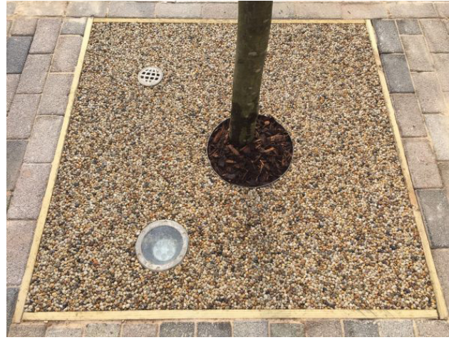
Figure 29- Resin bound gravel filled tree pit with bark mulch fill around collar and irrigation system embedded.
